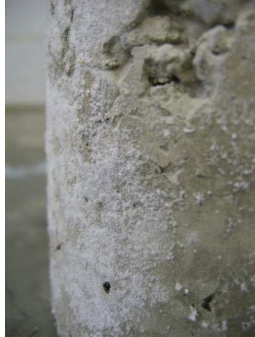
Figure 6. Efflorescence in GPC
