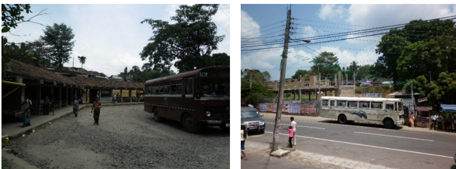
Karaliyadda- earlier bus station is demolished and a new modern type multi-storey bus station is in the process of construction.
