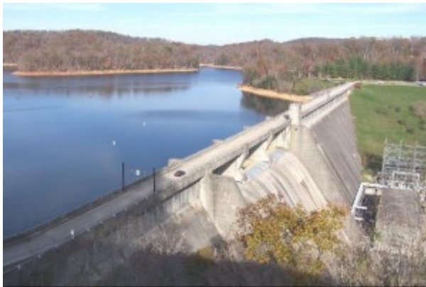
Figure 4.3 Norris Dam, United States. The First Dam Built by the Tennessee Valley Authority (J. Stephen Conn, flickr , accessed July 16, 2015, https://www.flickr.com/photos/jstephenconn/. )
