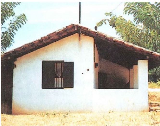
Figure 7.40 Experimental Core-House Built in 1984 by the MAU in Digana for Rs. 25,000 Using Mud Bricks with Cinnavan (photograph and description by Shanti Jayewardena in Jayewardena, "Mahaweli Development Programme", 39.)
