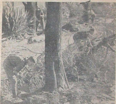
TODAY'S PICTURE of preparations for the building of the Bonython Great Hall at the University. The workmen are clearing the ground on the site of the building.
