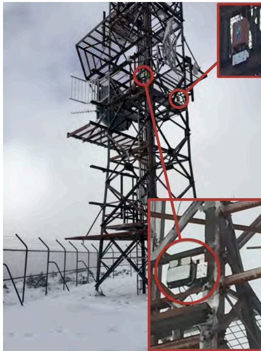
Fig. 5.2 Tower structure on which the holographic instrument and Polarsonde were deployed. A zoomed in view of the holographic instrument is shown in the bottom right inset and the Polarsonde is shown in the top right.
