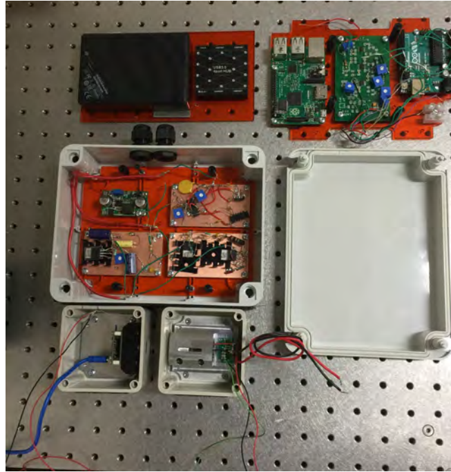
Fig. 4.21 Image of the final developed instrument before the boxes were sealed. Each of the electronic control stages can be independently adjusted and then all components are mounted within water proofed plastic boxes.
