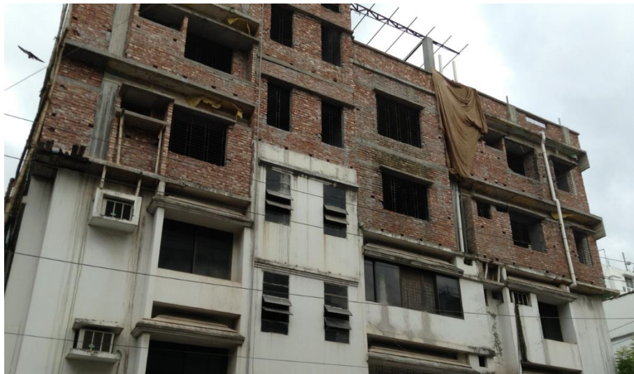
Figure 5.27: An Under-construction Building, Showing the Common Construction Materials and Practices. Source: Field Study
