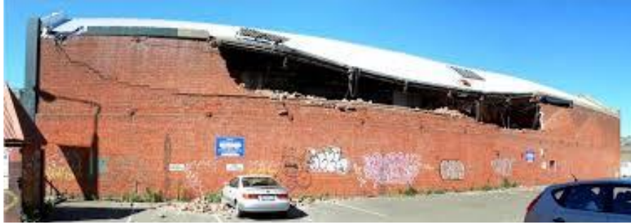
Figure 2. Out-of-plane wall failure caused by excessive diaphragm deformation (Dizhur et al. 2011)
