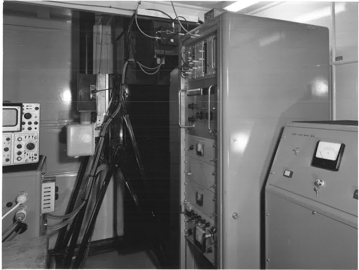
FIGURE 2.1 The laser radar equipment installed inside the mobile instrumentation van.
