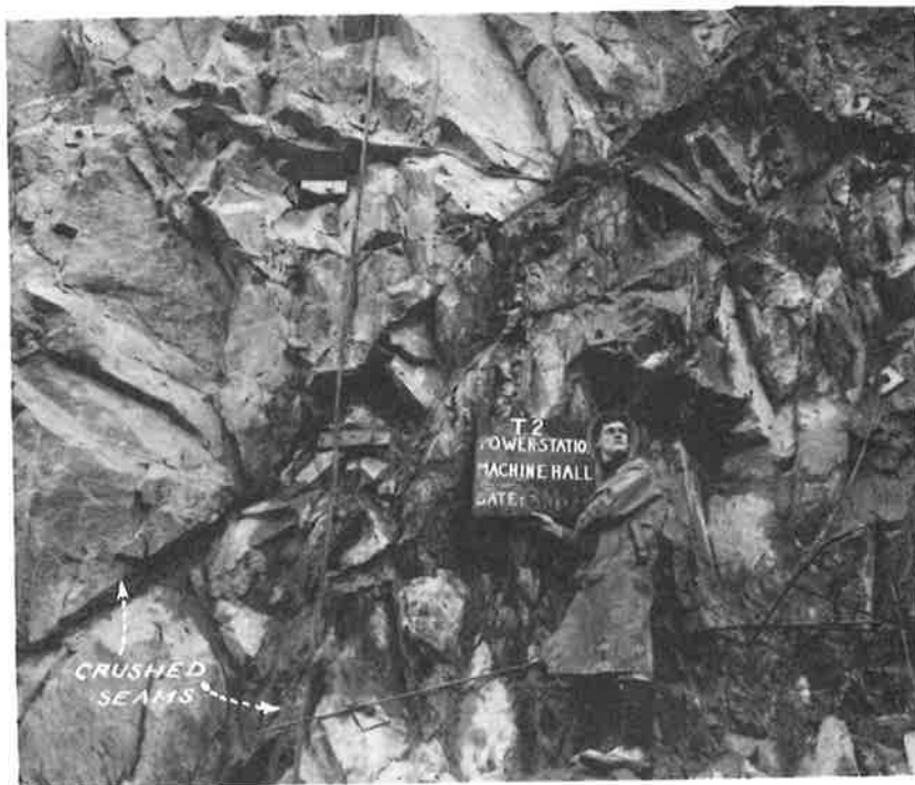
PLATE 16. Granitic gneiss at the Control Building end of the downstream wall. The rock has broken along joints and minor faults, rather than across its own fabric. Few traces of line drill holes remain.
