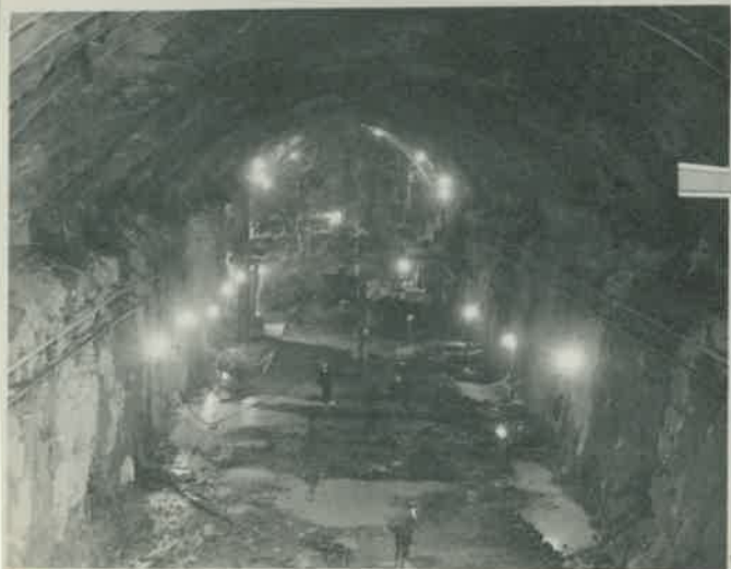
5 Deepening of excavation to 51 feet from roof and excavation of penstock and draft tube tunnels
