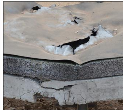
(c). Fractured cover plate and concrete
