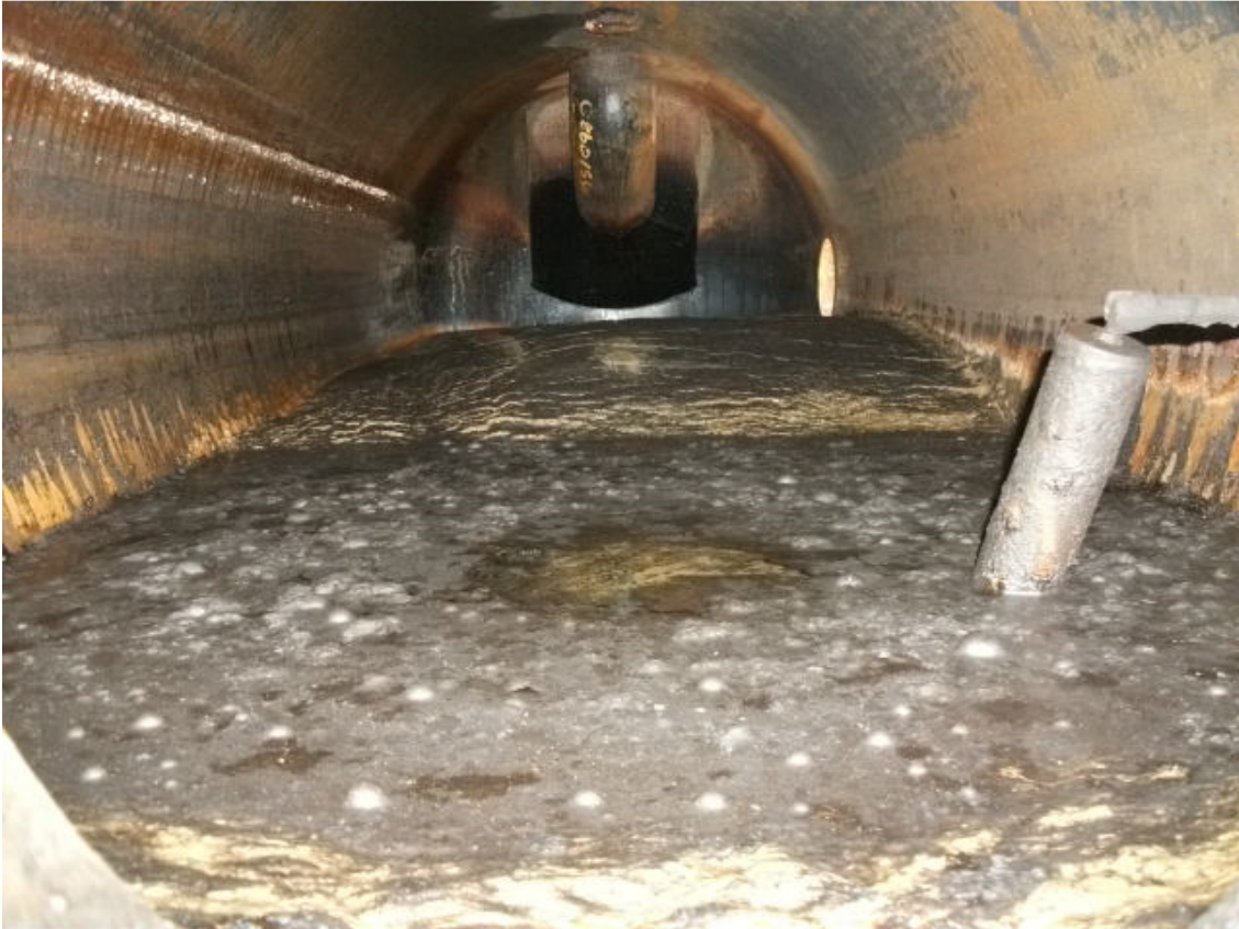
Figure 1: Fines produced from Condabri South 19 which has accumulated in the separator.
