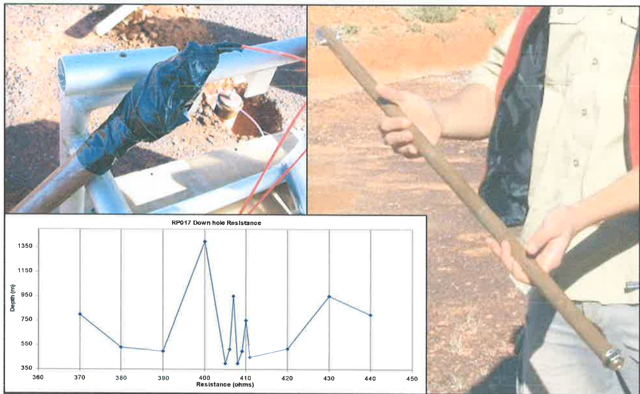
Figure 3.48: (top left) Shackle bound in electrical tape to reduce chances of snagging. (bottom left) Graph of resistances measured down-hole. (right) Prominent Hill electrode, 1m long, 20m diameter copper pipe with 20mm Dynabolt at the bottom and 8mm shackle at the top.
