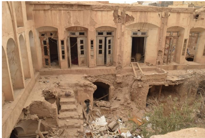
A dilapidated abandoned building in historic Kashan, 2018 (Source: author)
