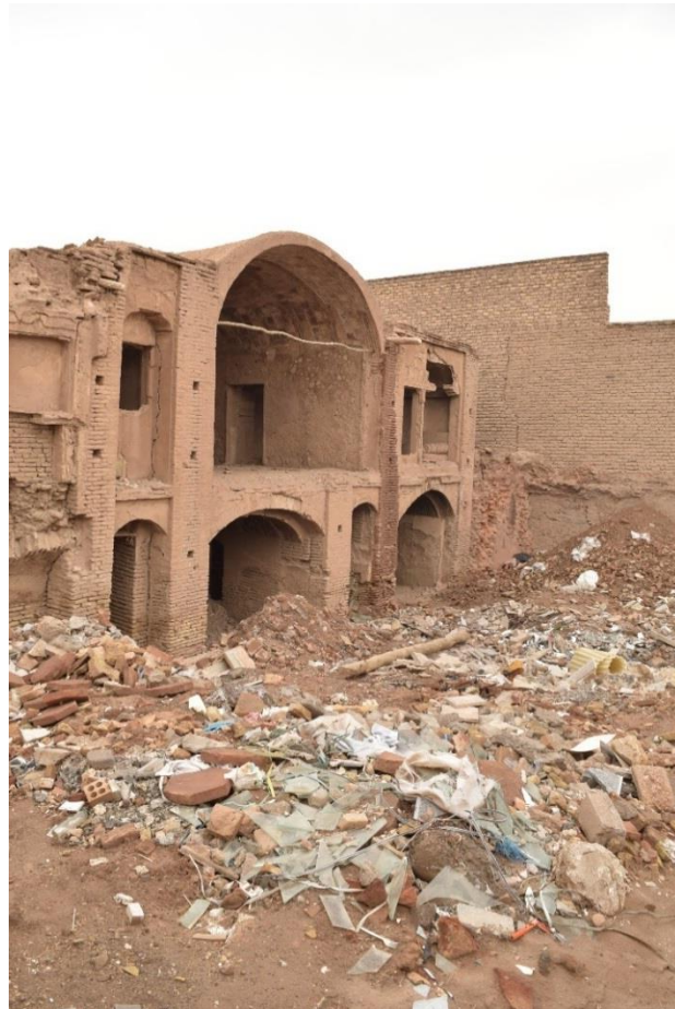
Dilapidated-abandoned building (DABs) in historic Kerman, 2018 (Source: author)
