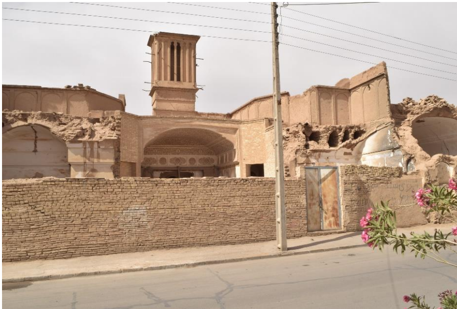
Figure 1.1: Today, historic cities are carved by new road developments that have turned traditional fabrics into disaggregated and fragmentary urban tissues (Yazd, Iran 2018), (Source: author)
