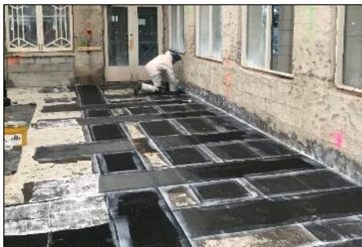
(d) Example of using FRP anchors to transfer the forces to the perimeter
