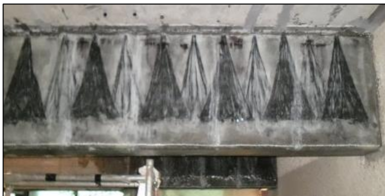
(c) Example of using FRP anchors to close the confinement of a coupling beam
