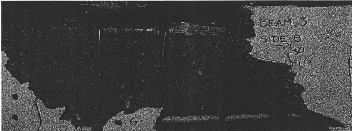
Figure 8.68. – Loose concrete removed from beam 3.
