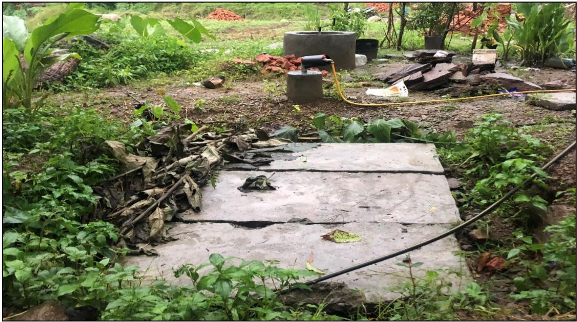
Figure 6.8 A newly constructed biogas plant in Sunder Bazaar
