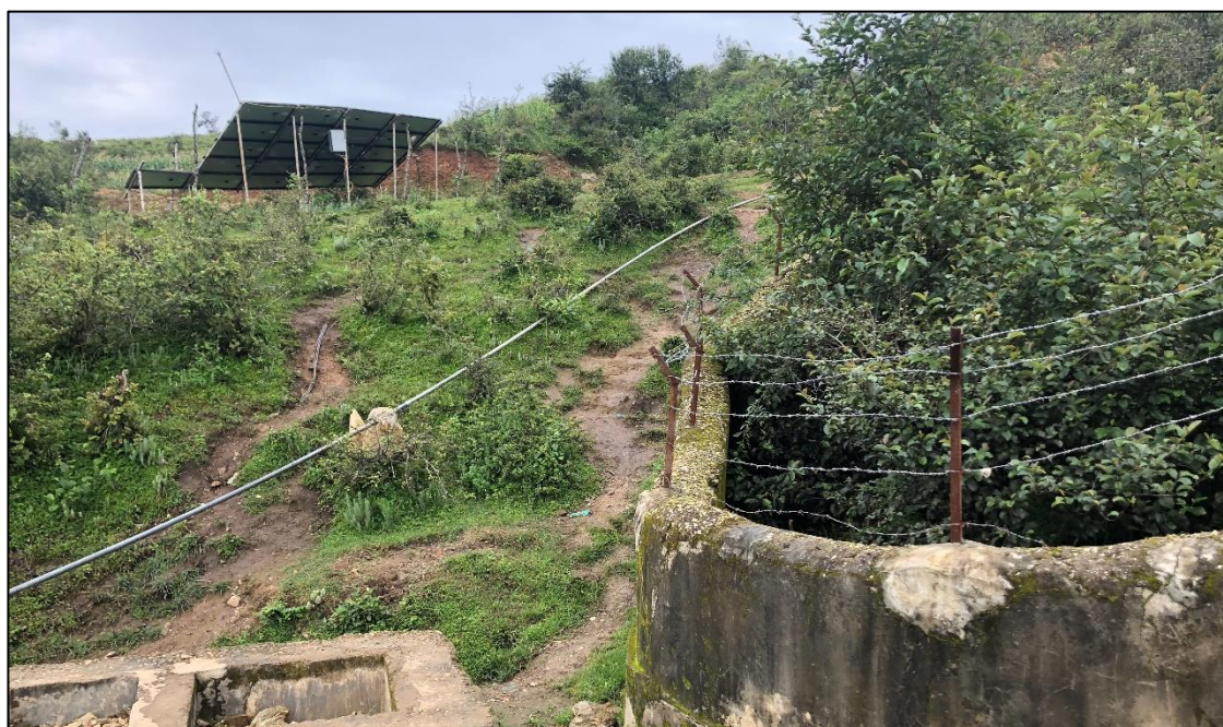
Figure 7.4 Solar PV based water pumping station in Kamal Bazaar
