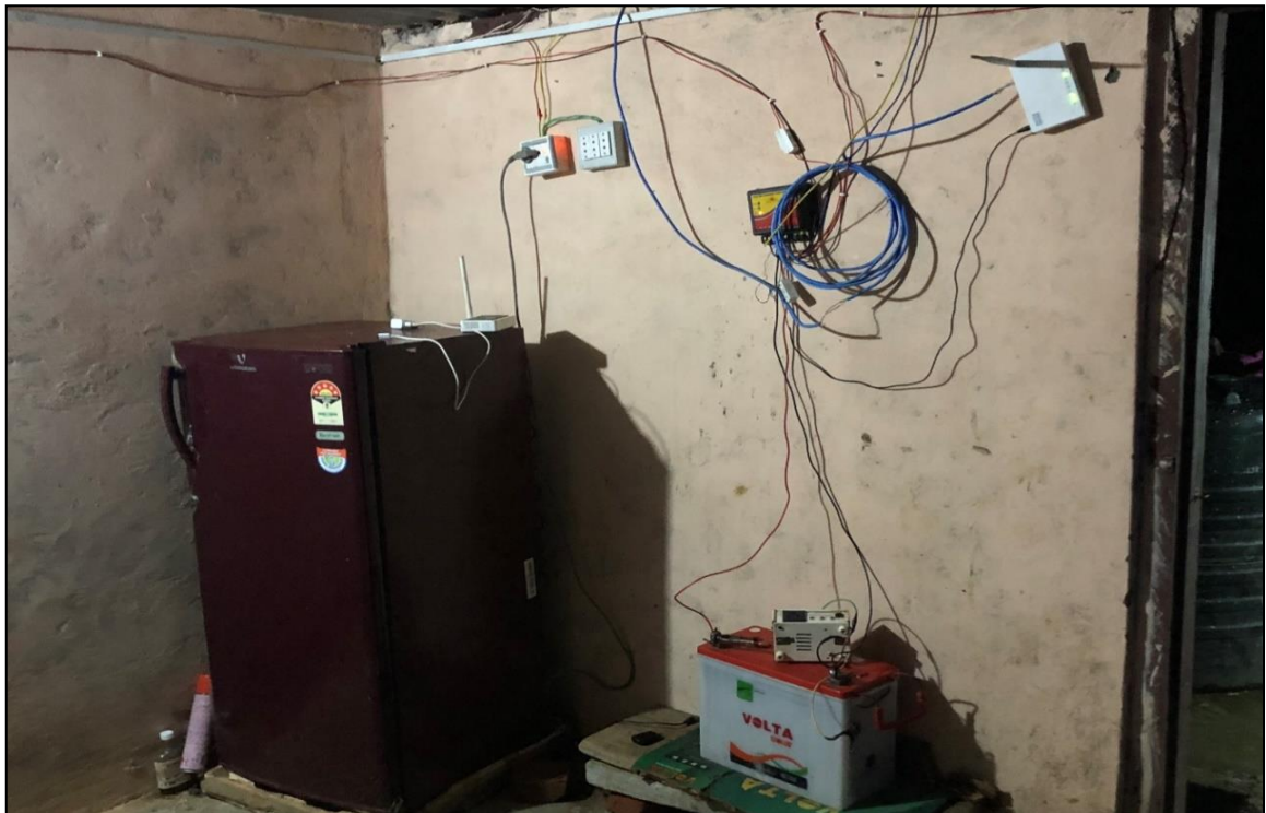
Figure 7.2 Refrigerator operating on a solar-wind micro grid power at a hotel in Kamal Bazaar
