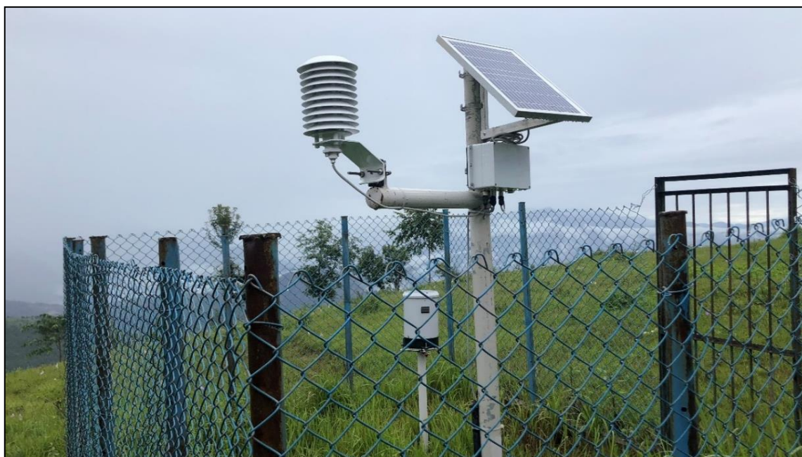
Figure 7.6 Solar PV based weather monitoring system in Kamal Bazaar
