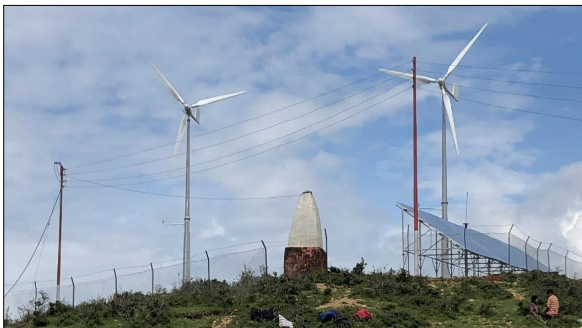
Figure 6.5 Solar-wind micro grid system in Kamal Bazaar, Achham
