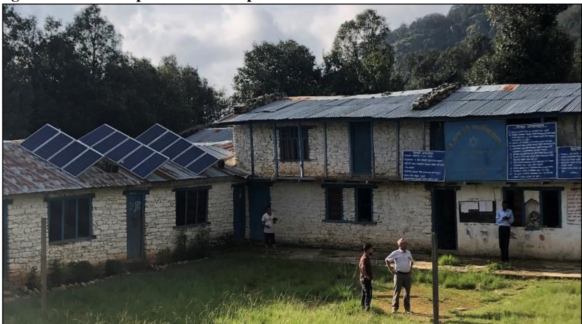
Figure 6.2 Solar PV panels on rooftop at a school in Kamal Bazaar
