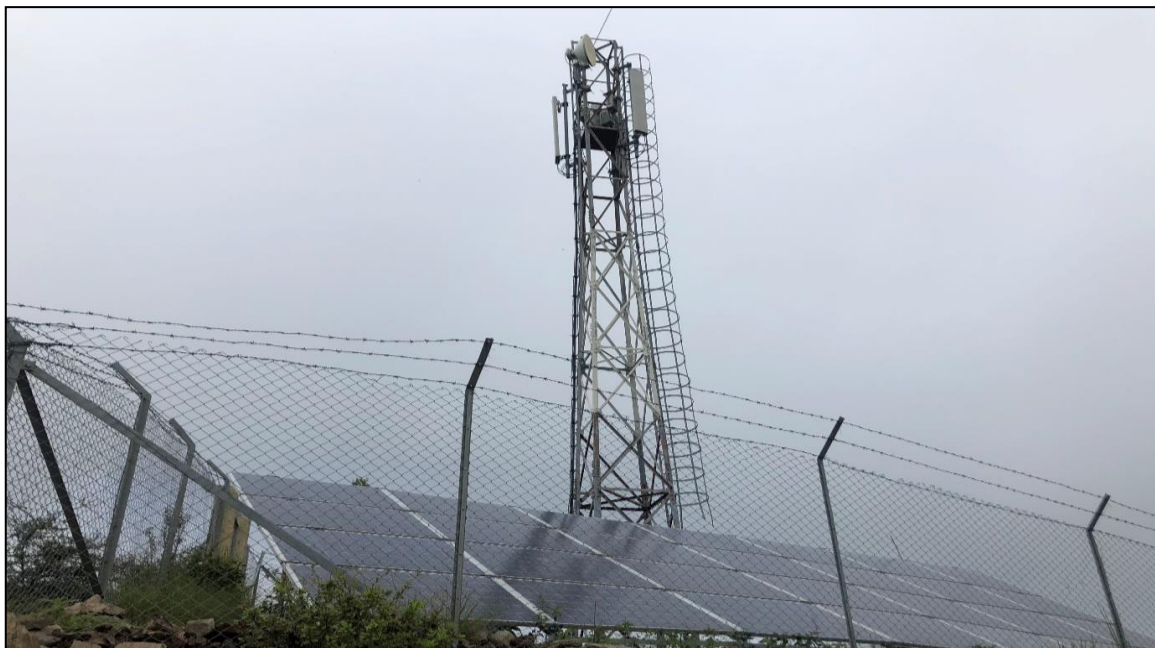
Figure 7.7 Solar PV based telecom infrastructure in Kamal Bazaar
