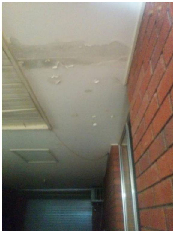
Figure 7. Leaking roof which is unsafe for children.
