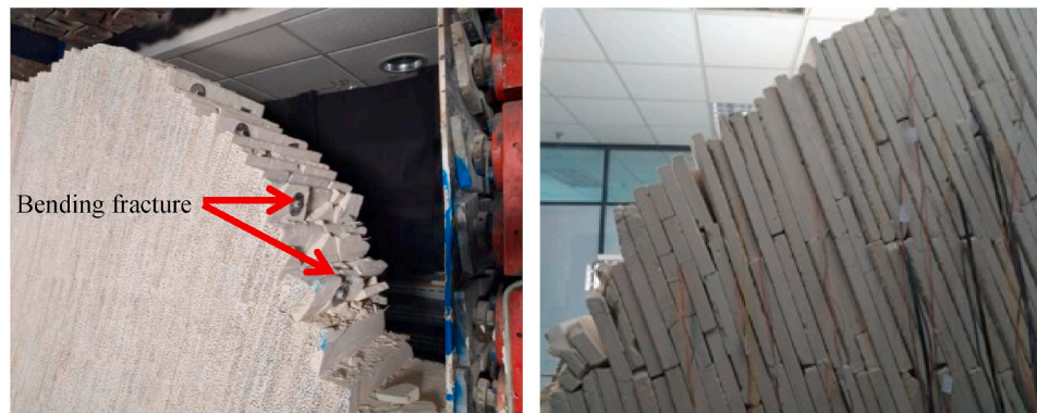
(b) Failure characteristics of the side of anti-inclined slope model reinforced by PR anchor cables
