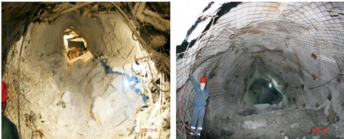
Figure 5.1 Rock ejection and deformation of the supporting system due to strainbursting (Feng et al. 2017)
