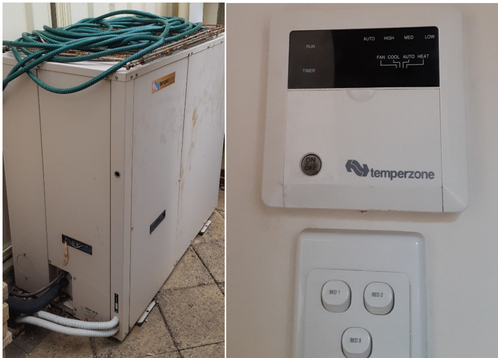
Figure 8-3 - House 08's HVAC system and controls. Source: Photographed by the author.
