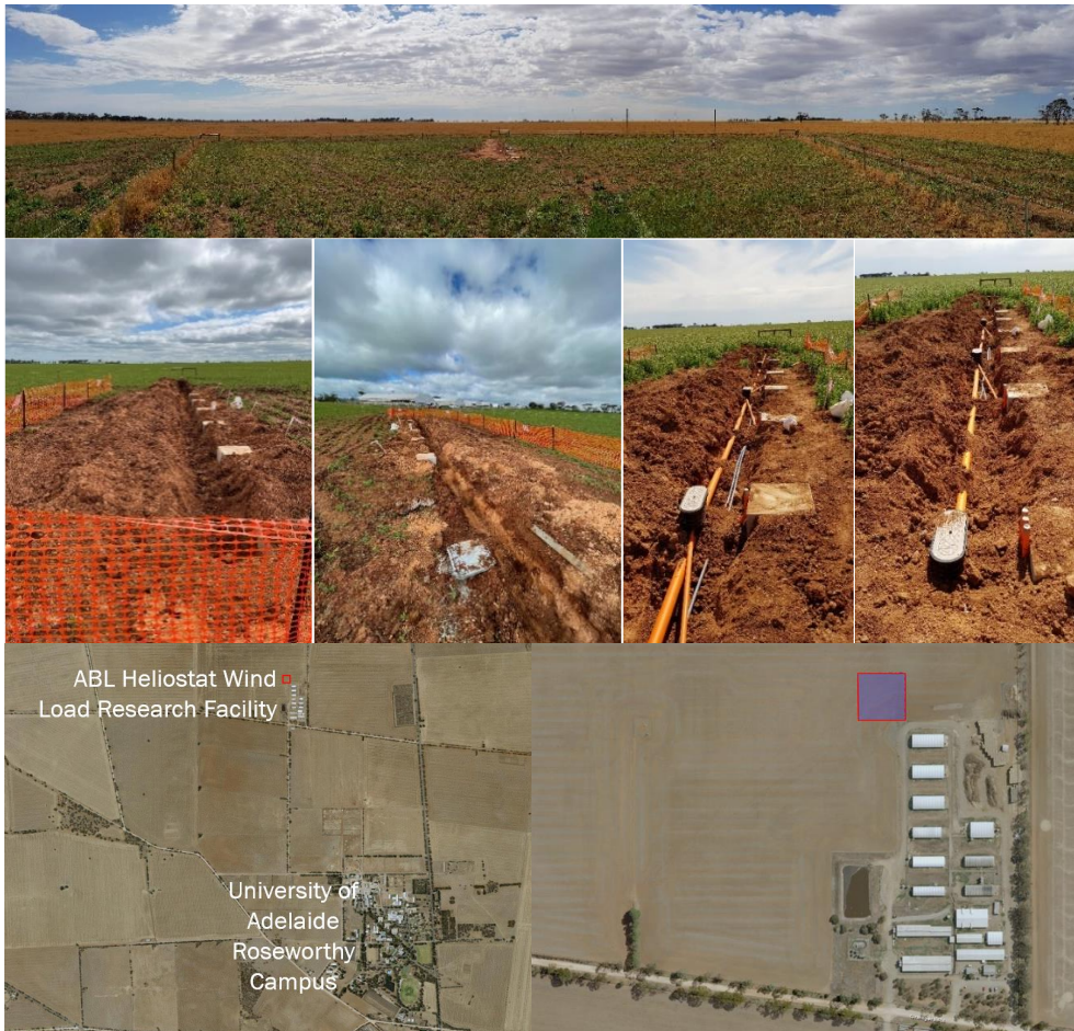
Figure 1. Site preparation stages including fencing, trench excavation, installation of mast foundations, water pipe and pits within the 50 m × 50 m fenced area of the Atmospheric Boundary Layer Research Facility (ABLRF) at the University of Adelaide Roseworthy Campus field site (34°30'37.0"S 138°40'37.3"E).
