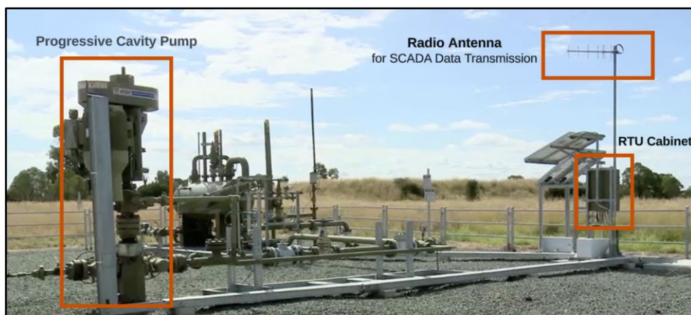
Figure 7 – CSG Well Layout depicting the PCP and RTU and Radio Antenna for data transmission.
