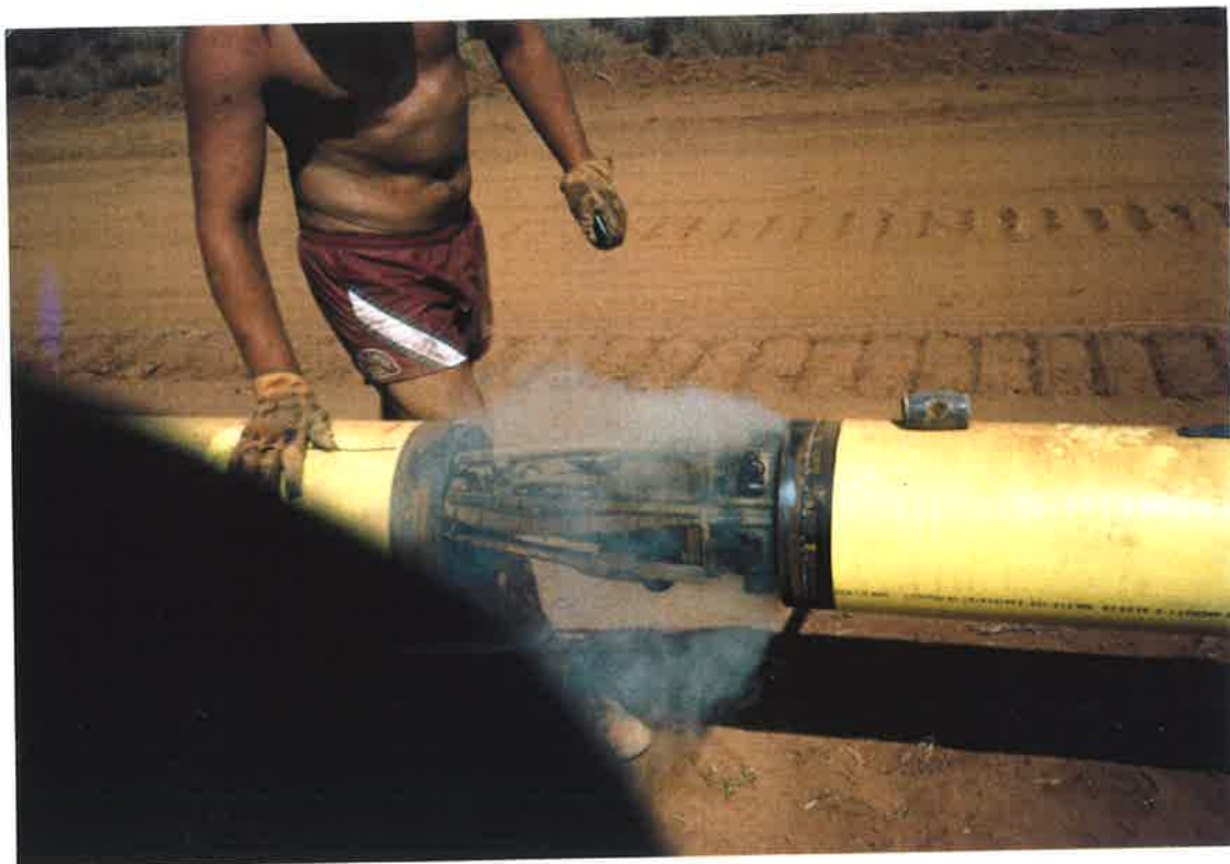
Figure C6: Photograph showing two pipes being brought together over the internal clamp. The pipe on the left hand side of the photograph is held and moved by a sideboom.
