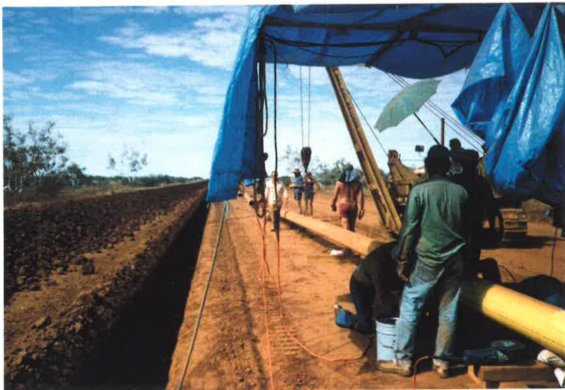
Figure C8: Photograph showing, in the foreground, the two front end welders working opposite each other and, in the background, the pipe being held by the sideboom.
