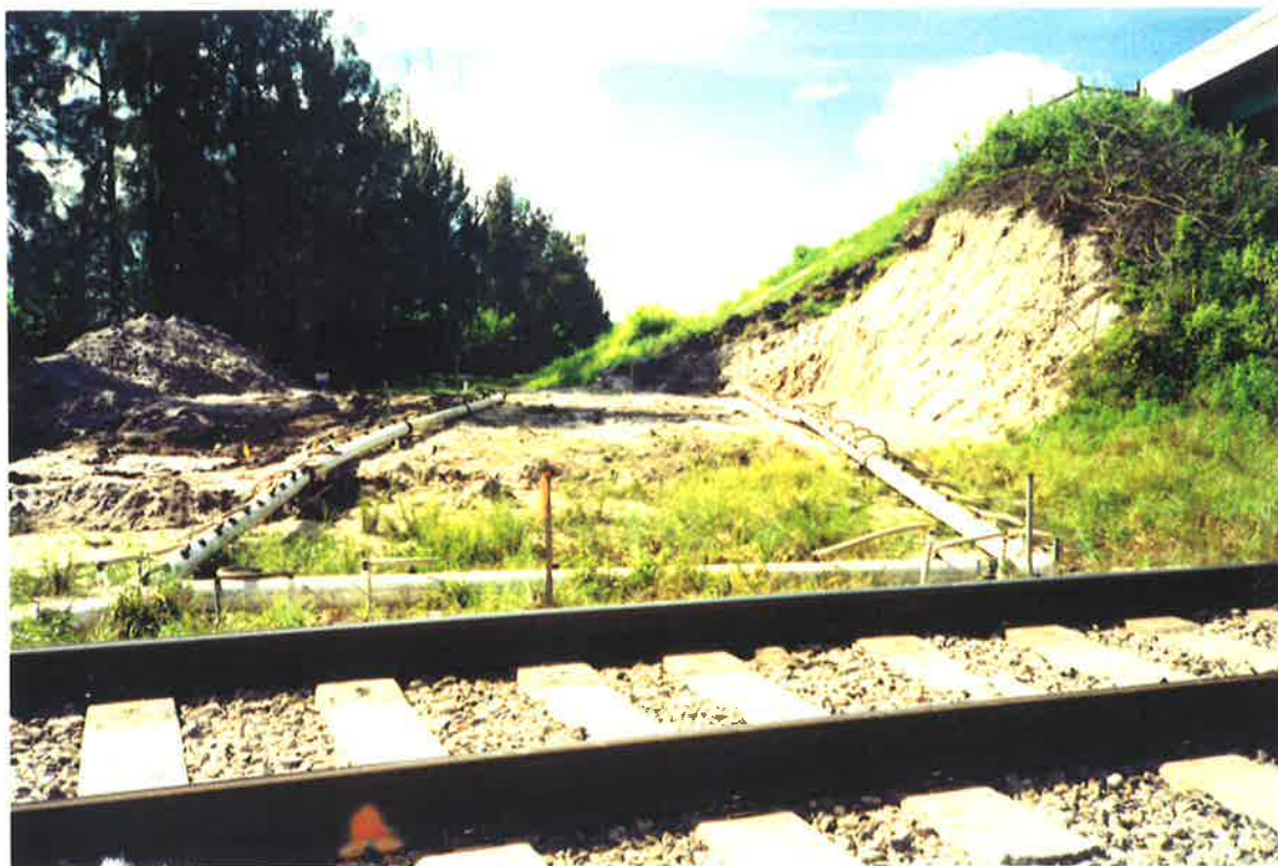
Figure C11: Water and sediment are pumped through pipes installed in the ground and through the ones above ground as seen in this figure. This particular area was being dewatered prior to boring operation underneath the railway tracks seen in the foreground.
