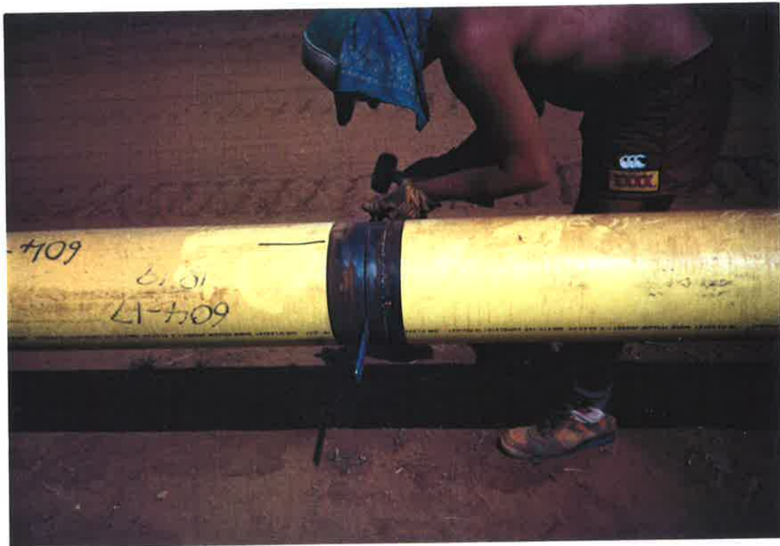
Figure C7: Photograph showing setting of the root gap using spacing tools (or spacers) which are hammered into the joint. The spacers are left into the joint until during the welding operation when they are removed.
