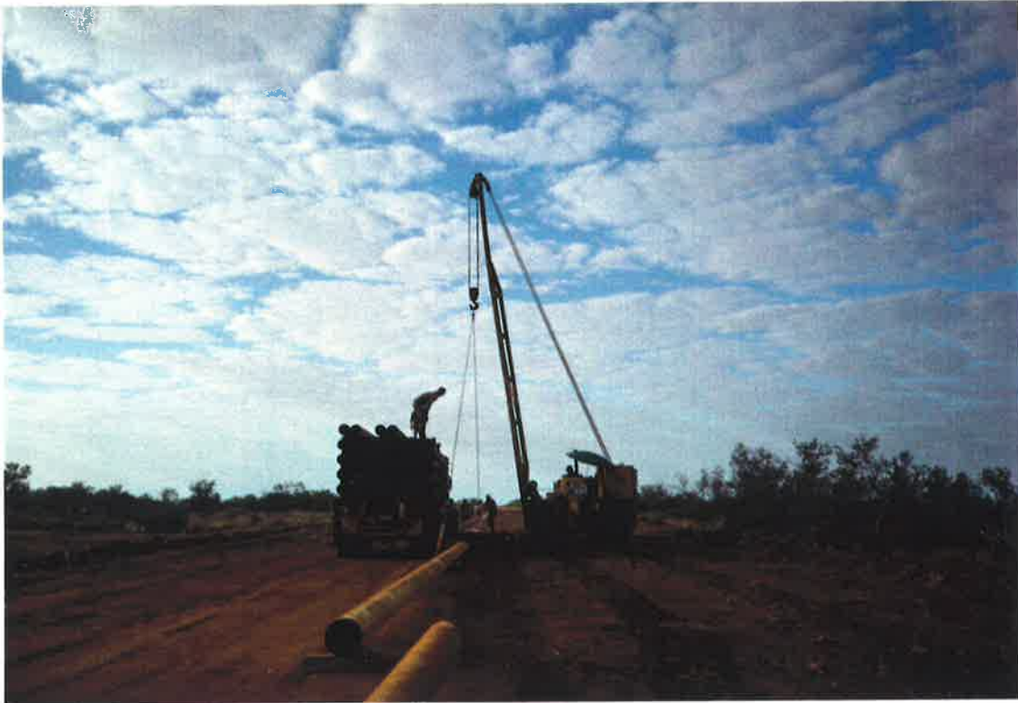
Figure C4: Photograph showing a sideboom lifting a pipe from the truck and laying it on the stiles.
