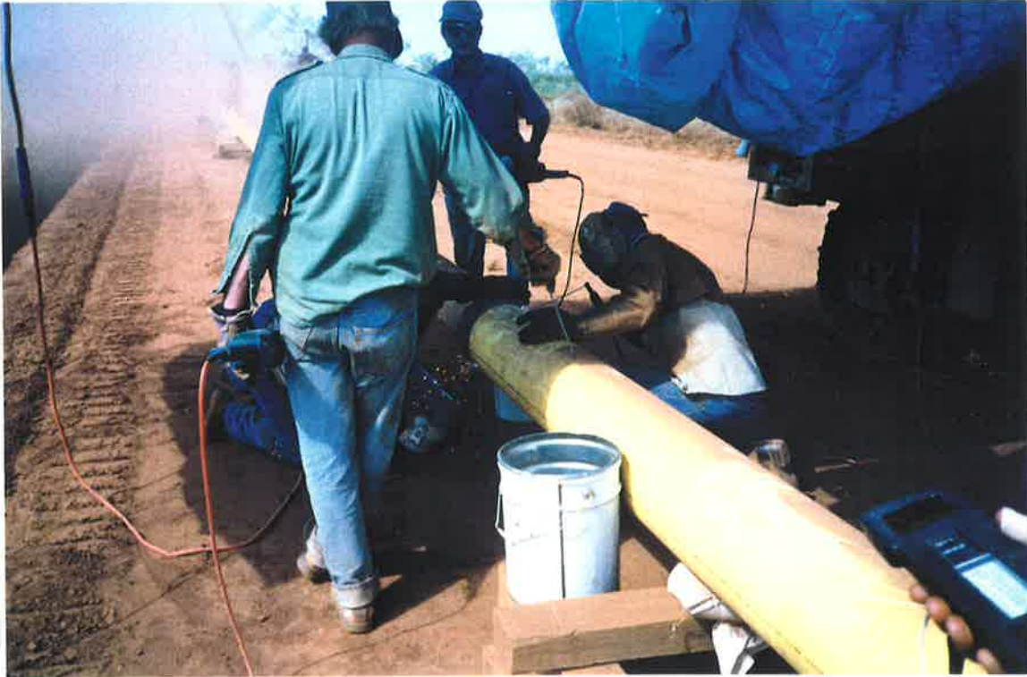
Figure C9: Photograph showing the two front end welders welding the root pass in more detail.
