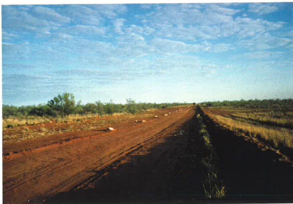
Figure C3: Photograph showing the right-of-way which is graded and cleared prior to digging the trench and laying the pipe.
