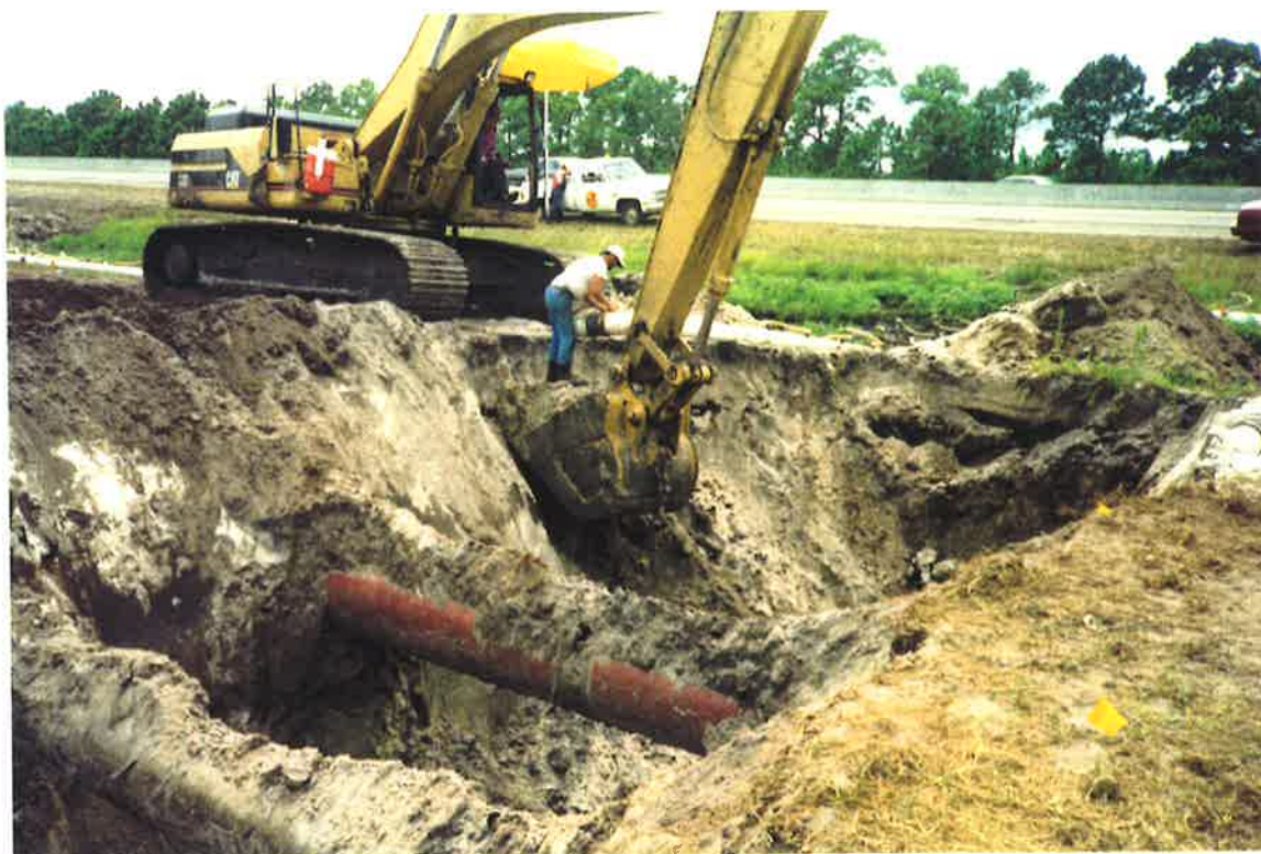
Figure C12: Digging of the trench with a back-hoe. The existing pipeline can also be seen.
