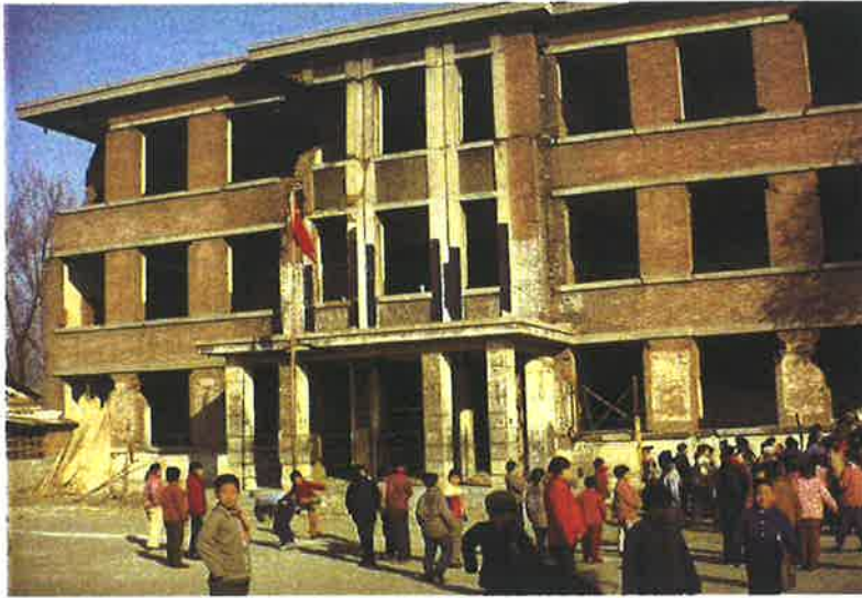
Figure 2.4.4 Damage to URM Building, Tangshan, China, 1976
