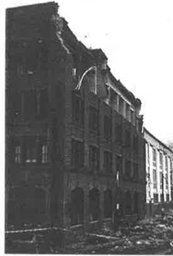
Figure 5.1.1 Out-of-plane Wall Failure during Loma Prieta Earthquake, 1989
