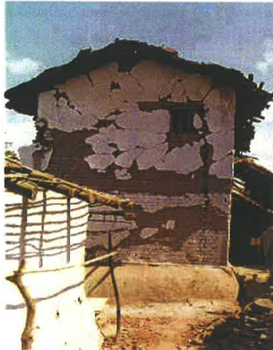
Figure 2.4.3 Masonry Damage During 1997 Jabalpar, India Earthquake (Jain et al 1997)
