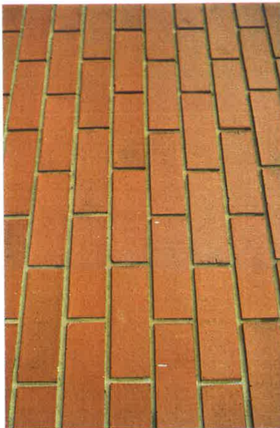
Plate 3-5 Tilted Photograph of Brickwork for Distortion Analysis
