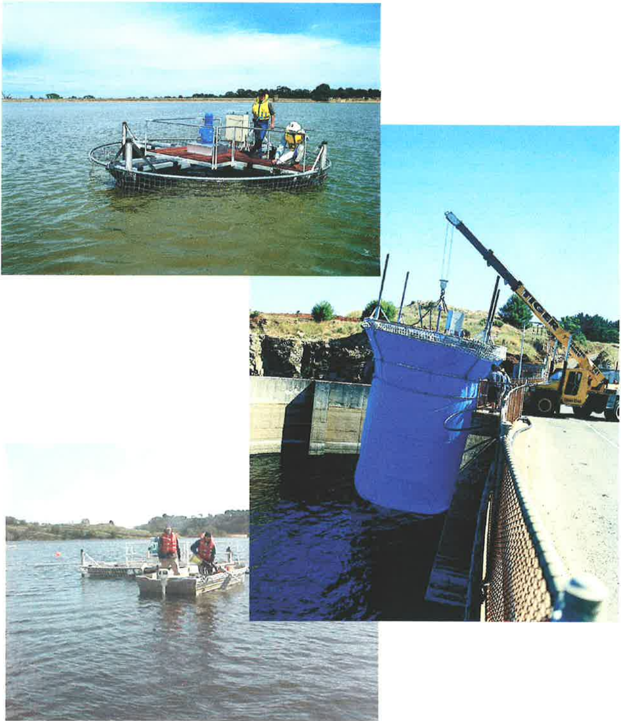
Figure 5.3 Photographs of the surface mounted mechanical mixer in the Myponga Reservoir, South Australia.
