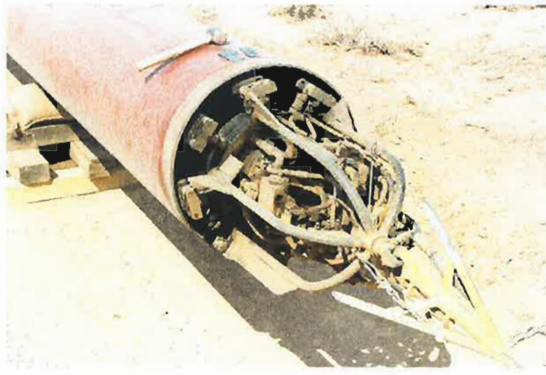
Figure 3.23: Photograph of a line-up clamp used to round and align pipe segments during pipeline construction.
