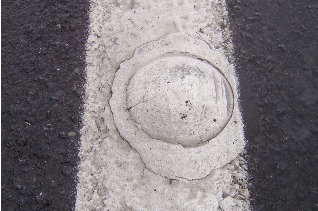
Figure 2.3 Close up of a Polydot on the Dukes Highway near Bordertown (source: J Woolley)
