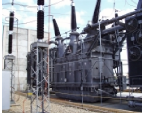
Figure 7.1 The test transformer
