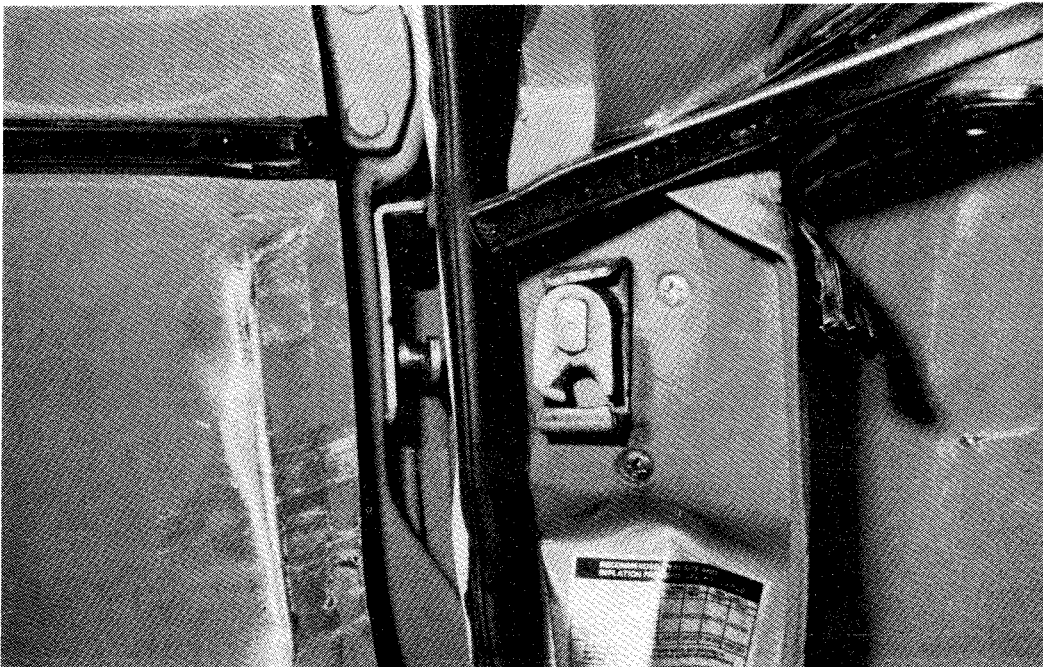
FIGURE 4.6: Separation of door latch without significant damage to the latch (see Fig. 4.5)
