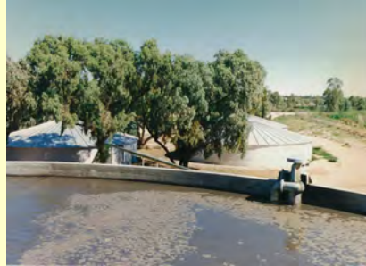
Treated Effluent Storage Tanks (background)
