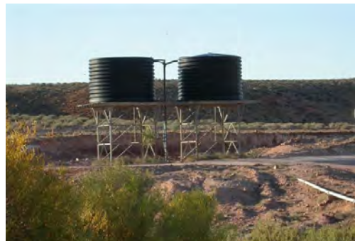
Storage Tanks at Blue Dam
