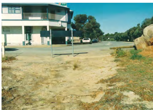
Stormwater Drainage Discharge
