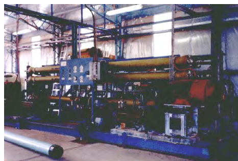
Reverse Osmosis Plant
