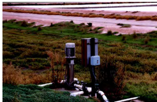
Irrigation Pumps (Rabone 1994)
