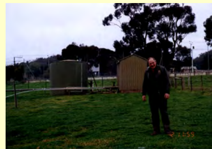
Storage and pump station
