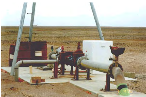
Raw Water Bore
