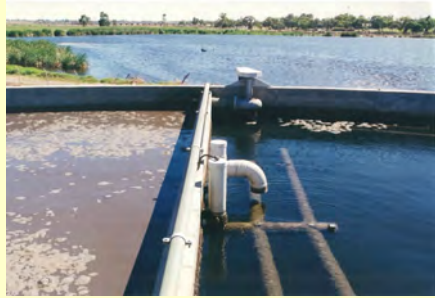
Treated Effluent (front right) & Emergency Storage (background)
