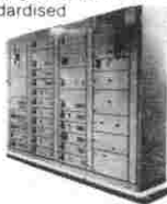
An ASEA VMG switchboard.
