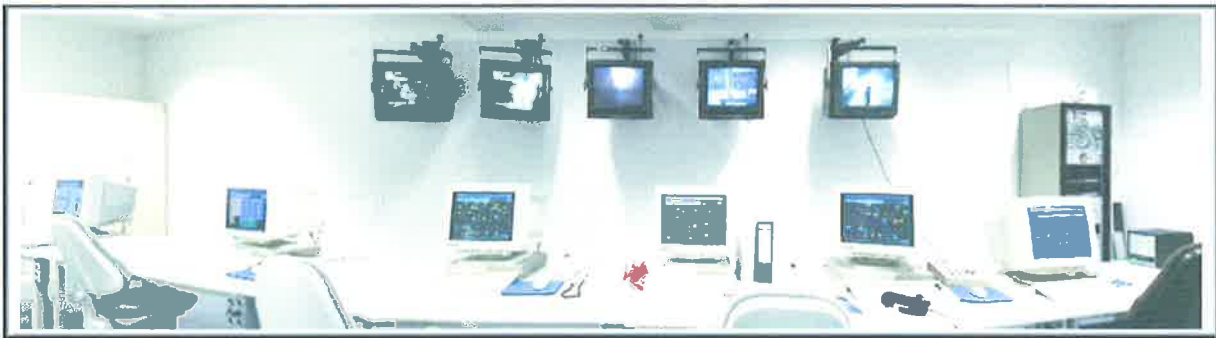
Figure 3.1 Remote operations in the control building (D68) for the P8 test facility
