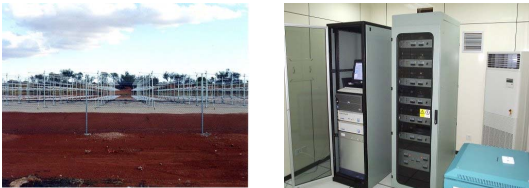
Figure 13 the VHF antenna array at Woomera (left), and Xian radar hardware.
