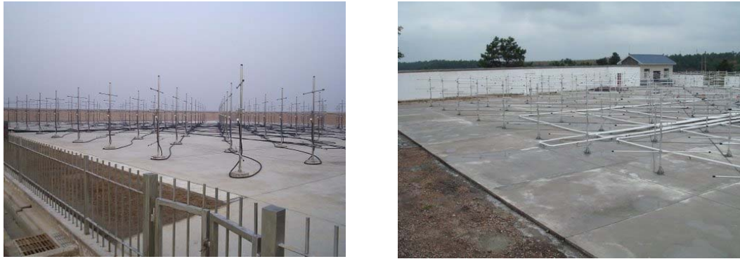
Figure 12 the VHF antenna array at Xian (left), and at Kunming, China (right)
