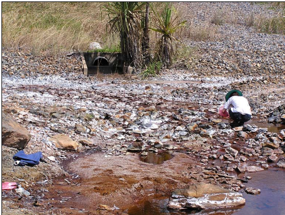
Plate 4.1. White efflorescence salts at Rum Jungle site RJI1.
