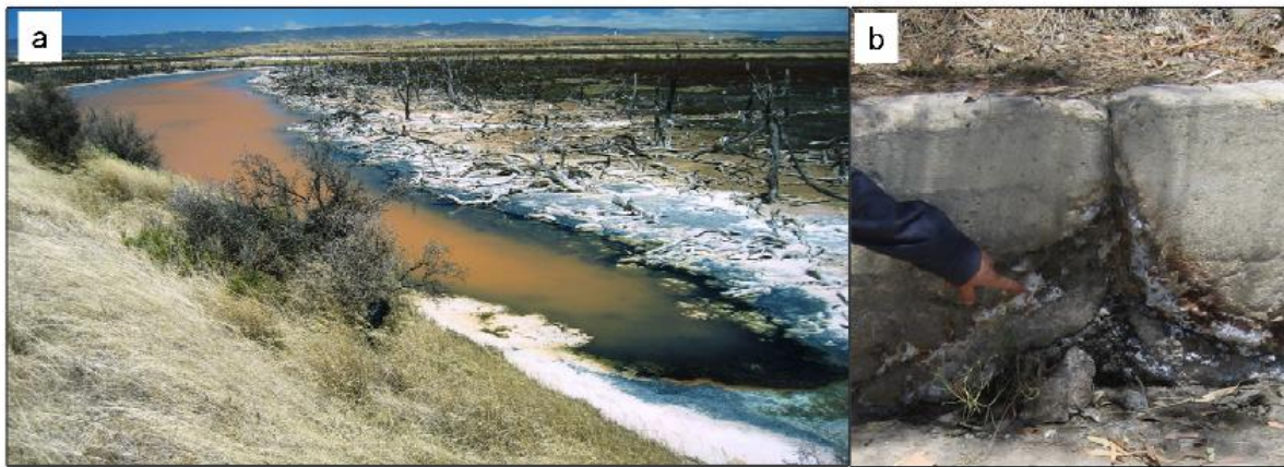
Figure 2-3 (a) stranded tidal creek at Gillman with water containing orange iron oxyhydroxide and surrounded by white salt deposits and dead mangrove tree stumps. This site has low aesthetic characteristics. (b) corroded concrete drain at Gillman.
