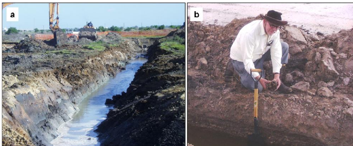
Figure 10-3 (a) and (b) excavation of experimental drain (16 th August 2002) in acid sulfate soil with sulfuric material and hypersulfidic material to investigate changes in geochemical and mineralogical processes as part of a series of management trials in the Gillman Focus area A. Image (a) shows a drain excavated in sandy soils typical of map unit 5 (e.g. soil profile BG 15) and 6 (e.g. soil profile BG 11). Image (b) shows Prof. Delvin Fanning holding a sample of sulfuric material exhumed from a drain in salt scalded mud flats, typical of map unit 3. The drain wall depicted in image (b) was described as soil profile BG 17.
