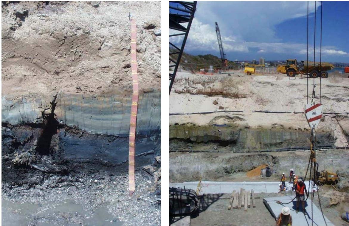
Figure 12-1 (Left image) Soil pit (Profile BG 2) at Gillman, Port Adelaide showing about 110 cm of calcareous clayey dredge spoil, used to raise the land surface, overlying 40 cm of sapric hypersulfidic material (derived from a former mangrove swamp) and underlain at 150 cm by coarse shelly material (chenier). This is a proposed new subgroup; Sulfic* Xerarents (Soil Survey Staff 2010). (Right image) Deep excavation at Barcoo Outlet, Adelaide (connecting the Patawolonga with the sea), and construction site through a sand ridge showing a relic hypersulfidic material buried under beach dunes (from a former mangrove swamp).
