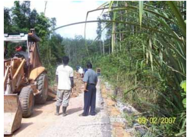
Pipe for water supply Construction along Jalan Jelawat Pos Iskandar, Tasek Bera
