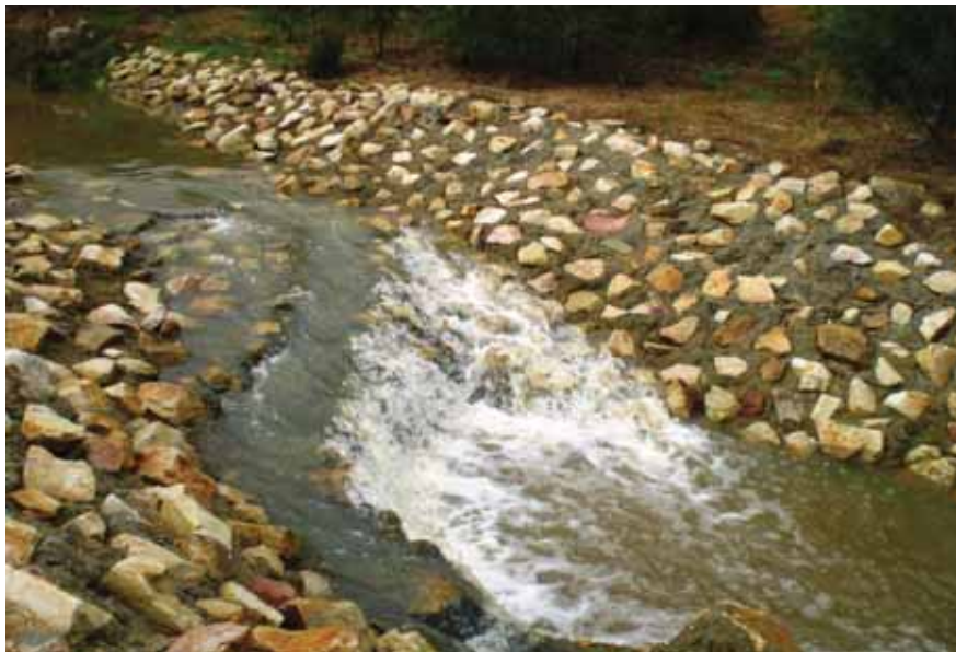
Figure 2.7: Photo of construction of concrete weir from the offline Brookes Bridge sedimentation basin. Note that similar construction of a concrete weir within Woodhouse Wetland allows water to bypass the wetland during high flood levels.
