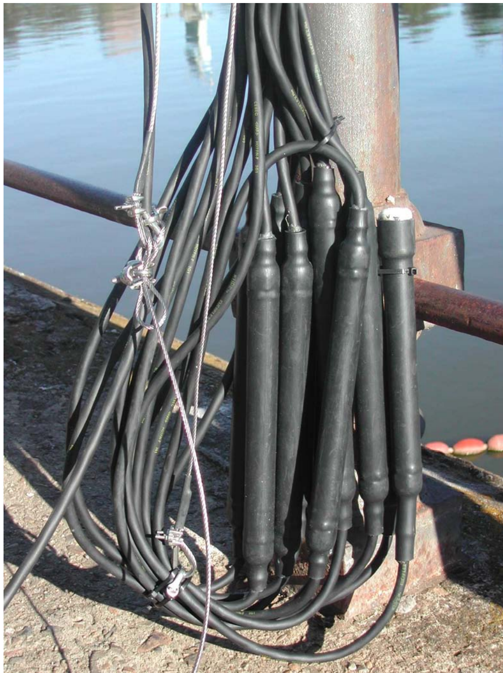
Figure 21 A sensor string bundled together for two-point in-field calibration at the Torrens Lake in Adelaide South Australia
