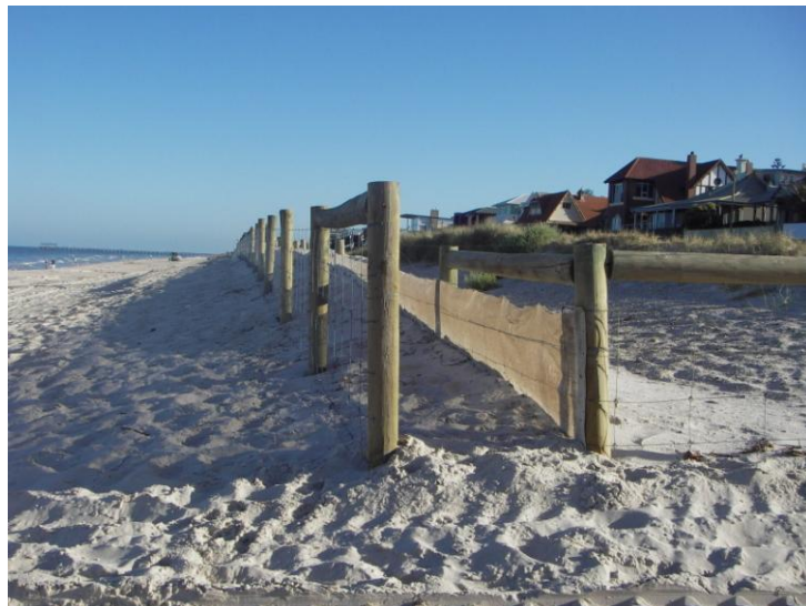
Figure 6.5. New fence being constructed seaward of existing drift fence used in this study. Photograph taken in February 2007. Source: Photograph by the author.
