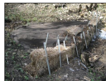
Figure 4: Overflowing sediment barrier trap
