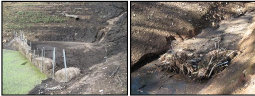
Figure 2 (LH) Algal growth adjoining hay bale sediment trap Figure 3 (RH) Destroyed trap on steep slope
