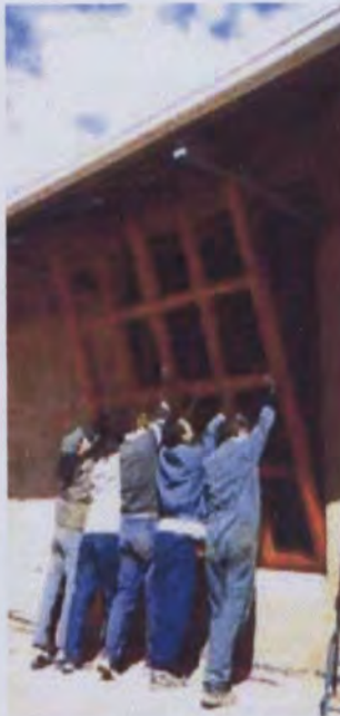
FIGURE 129: The Buddhist volunteers putting in place windows made by themselves from recycled timbers. (Muhlhan)
