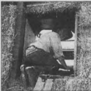
Ecopolis architect Paul Downton works on a window of the Whyalla Buddhist Meditation Group's EcoCity building.
