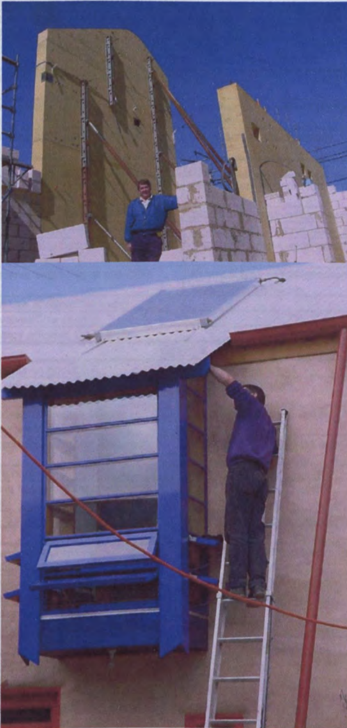
FIGURE 158: (top) Owner Michael Pilling with townhouse #2 under construction, showing mass walls of earthcrete and Thermalite blockwork (white). (below) EcoCity Development's Ian Rundle applies non-toxic 'Bio Products' paint to small bay of the Roman Hut. The blue was chosen by Roman's 8 year old son, Dylan. (Photos by author)
