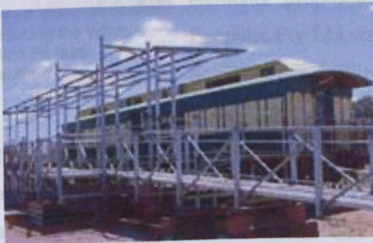
FIGURE 139: The refurbished, relocated railway carriage stands as a slightly uncomfortable reminder to many of some early miscalculations in planning for the EcoCity core site. (Photo by author)
