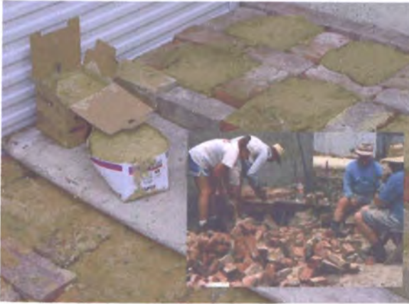
FIGURE 244: Resource recovery and reuse practised on the Christie Walk project. The bricks are from demolished structures on the site and will be used for paving – here they are also used to form moulds for paving slabs made from ‘waste’ concrete that otherwise would have gone to landfill. (Photos by author)
