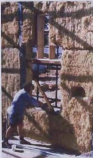
FIGURE 125: Strawbale walls under construction. Note niche carved in bales prior to cement rendering.
