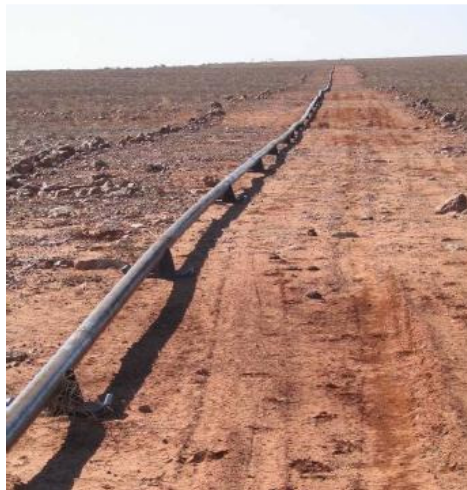
Figure 1.1: Typical aboveground pipeline in Australian outback
