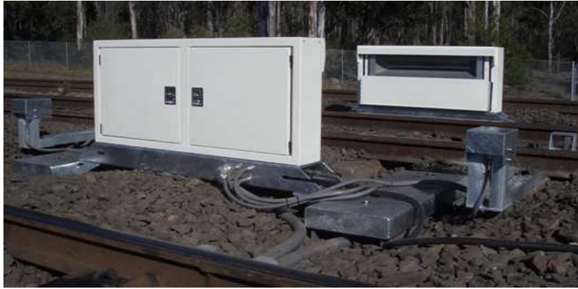
Figure 1.1: A photo of the RailBAM ® system [10] showing the wayside cabinets along with a few sensors (courtesy: Track IQ TM [11]).
